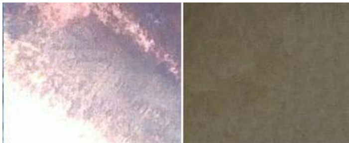
Before- flash rust
