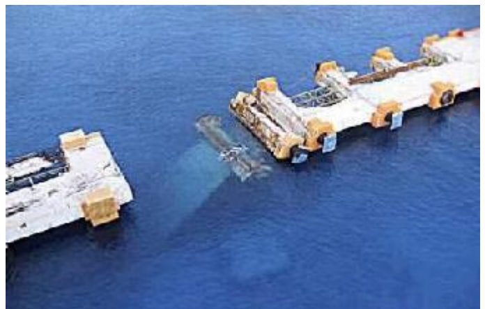
Cozumel Pier damage; note that clear water!
