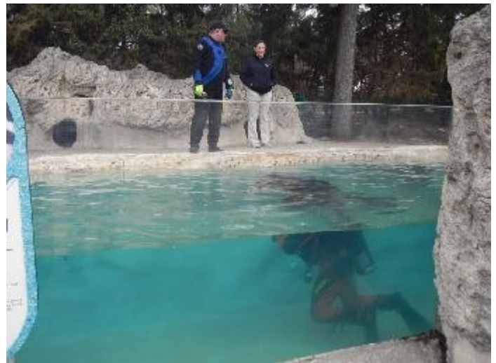
Dave works to replace a water jet as Greg and Robin Care, Children's Zoo Education Supervisor, look on.
