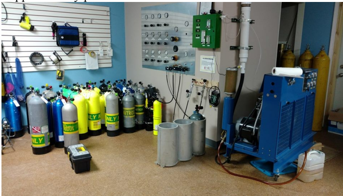
UWA compressor room with new boom boxes?
